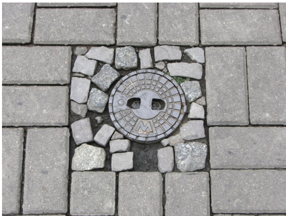
Regular surface box installed in pavement
